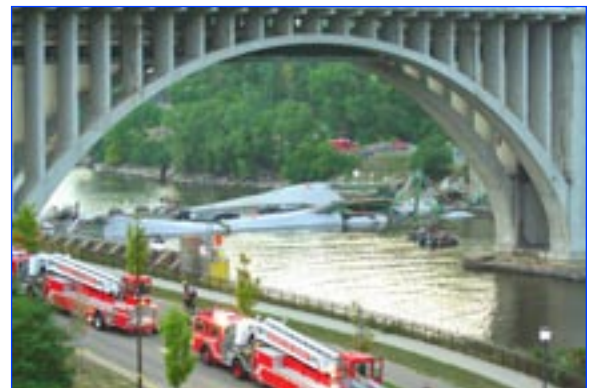
Emergency crews rush to rescue motorists on the collapsed I-35W bridge in Minneapolis. Photo by Poppysed Bandits.
